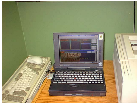
Figure 3. Network Service Center control computer
